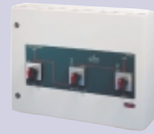
External Service Bypass Panel
